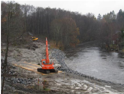
Building of a nature like by-pass channel at Hedefors power plant in River Sävån in October 2012.
