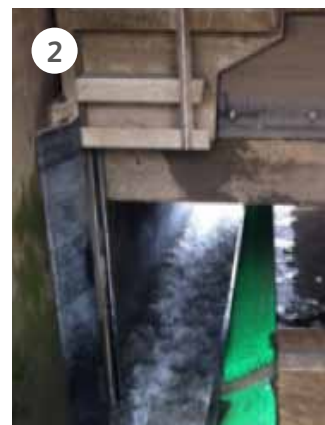
(2) One of the culverts and associated flap gate to be modified © Environment Agency copyright and database rights 2013
