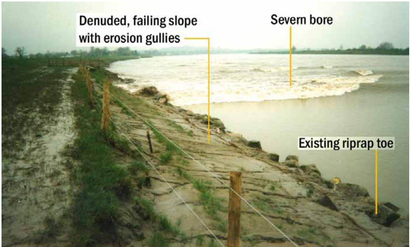
Eroding banks at Longney
