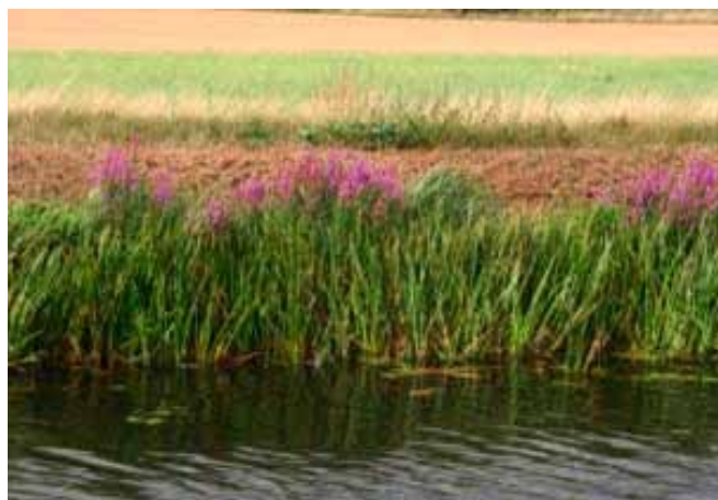
August 2011, new vegetation, branched bur-reed, has become established in front of the coir rolls ensuring the revetment process are naturally regenerating.
