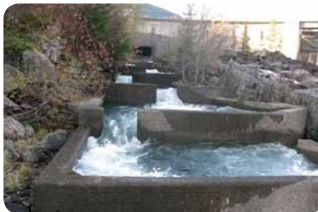
Point rehabilitation of secure fish migration past hydroelectric installation. (Odd Terje Sandlund, Norwegian Institute for Nature Research).
