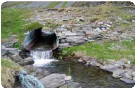
Point rehabilitation for stream continuity and fish migration: improvement of culvert pass under road filling. (2 photos before and after). (Knut Aune Hoseth, Directorate for Water Resources and Energy).
