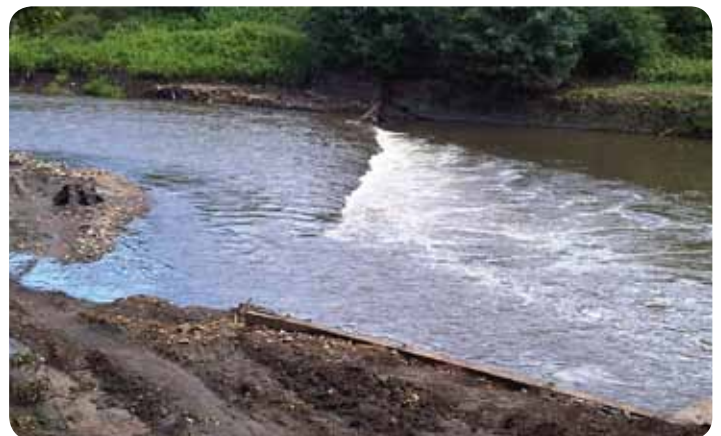
After initial completion of works (small bit of tidying to still do)
