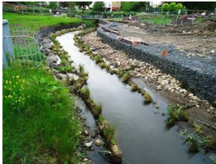
Channel restoration in Anderson park during works. Gabion baskets installed to constrain lateral channel migration. Photo courtesy of Gareth Greer - Rivers Agency (Northern Ireland).
