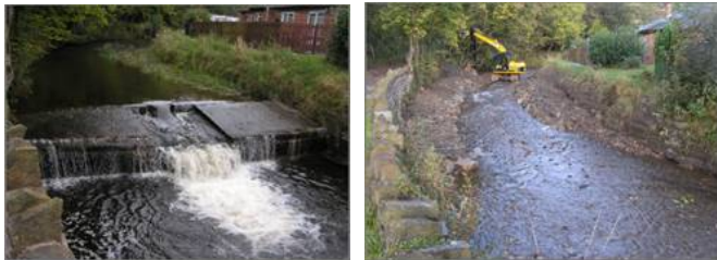
Before and after photos of weir removal – removal of redundant weir on River Irwell at Limy Waters
