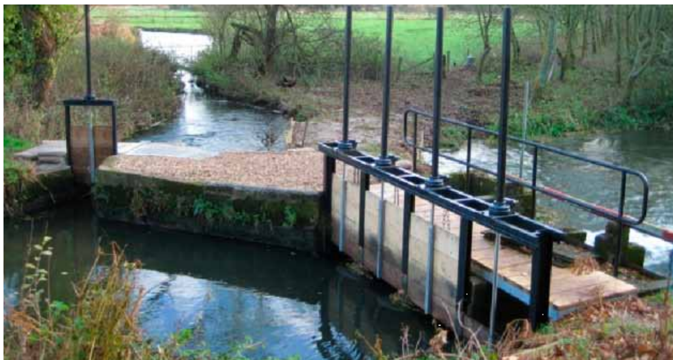
Hyford Hatches: restored allowing more effective and safe water level management through operation control.
