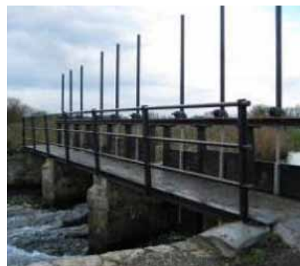
Water level control structures
