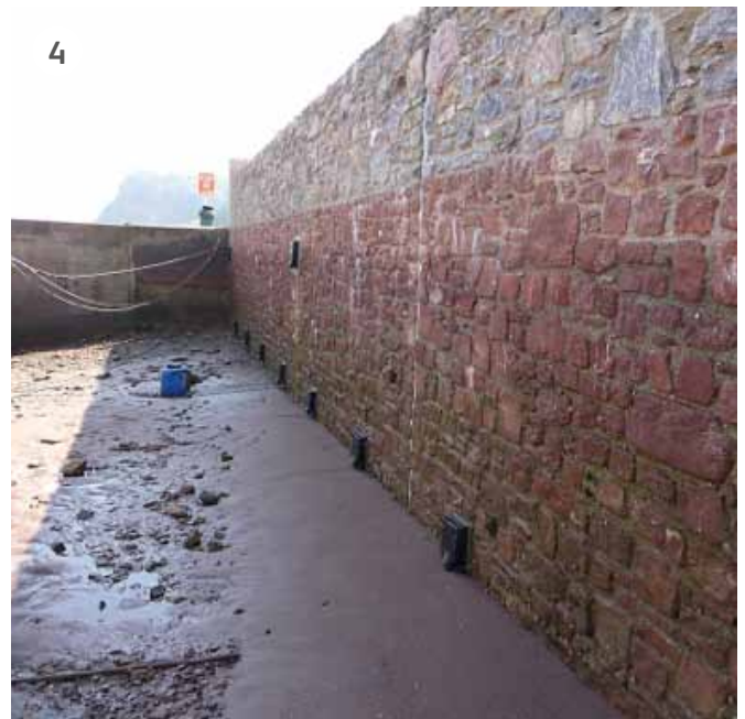
(4) New flood wall with ecological enhancements. Note low visual intrusion
