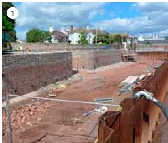
(1) Construction of two walls of the Shaldon and Ringmore tidal defence scheme, into which ecological enhancements were incorporated. May 2010
