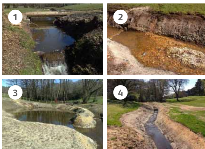
(1) Weirs creates acoustic feature along channel. Increasing in-channel morphological diversity; (2) Natural riffles forming. Increasing in-channel morphological diversity; (3) Online pond/ Backwater. Ecological value of marginal aquatic habitat, banks and riparian zone improved; (4) Two stage channel enhances ecological value of marginal aquatic habitat, banks and riparian zone.
