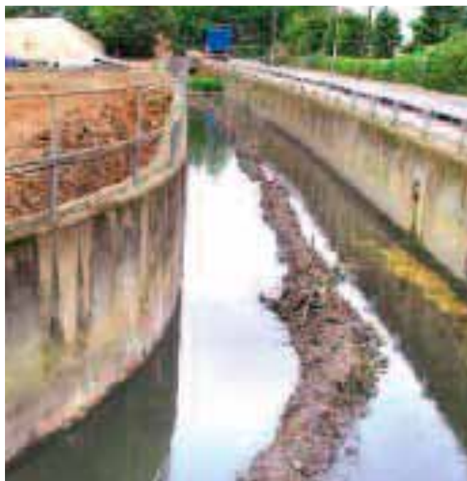
Pre-development 2004 - an unappealing drain All photos © Environment Agency copyright and database rights 2013
